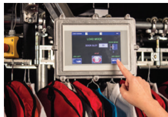
Loading station touch screen
